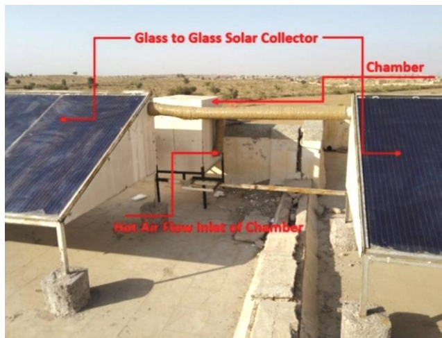
Fig. 1 — Hot Air dryer of glass-to-glass module.
